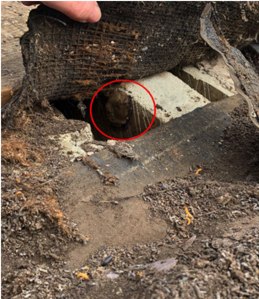
Pipistrelle bat below roofing felt.
