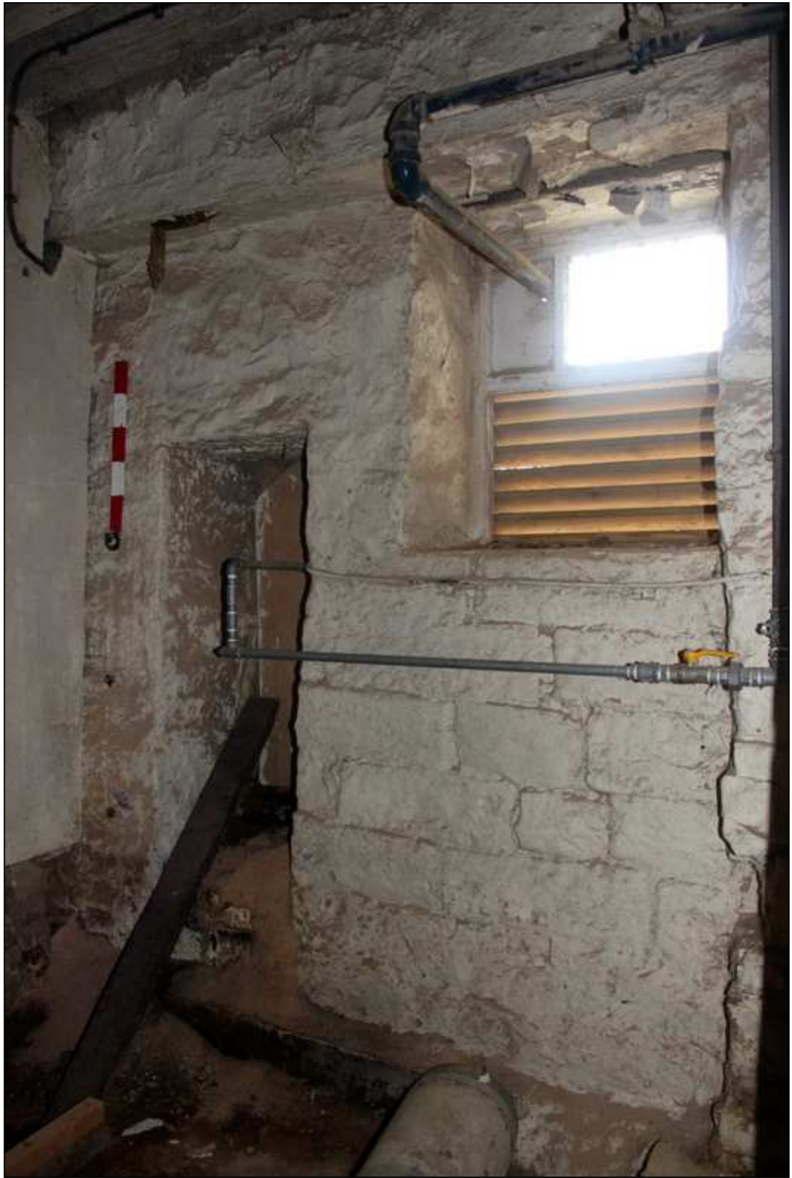
Plate 44: Blocked aperture in the south wall of the engine house, with possible bearing box on the left
