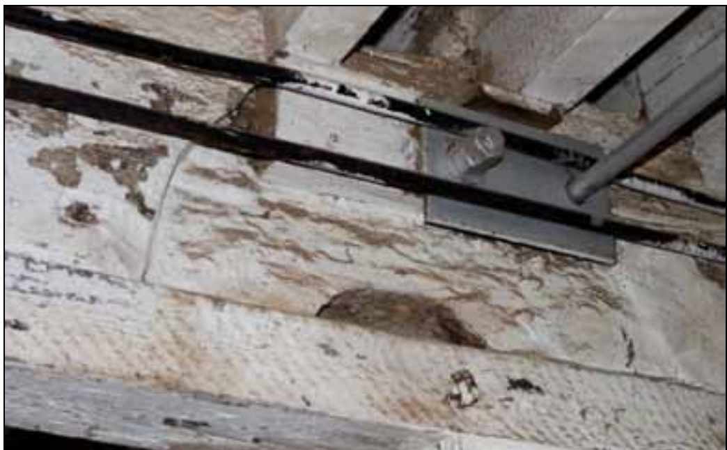
Plate 52: Rebate for drum on original line shaft, with cut-out in soffit for shaft
