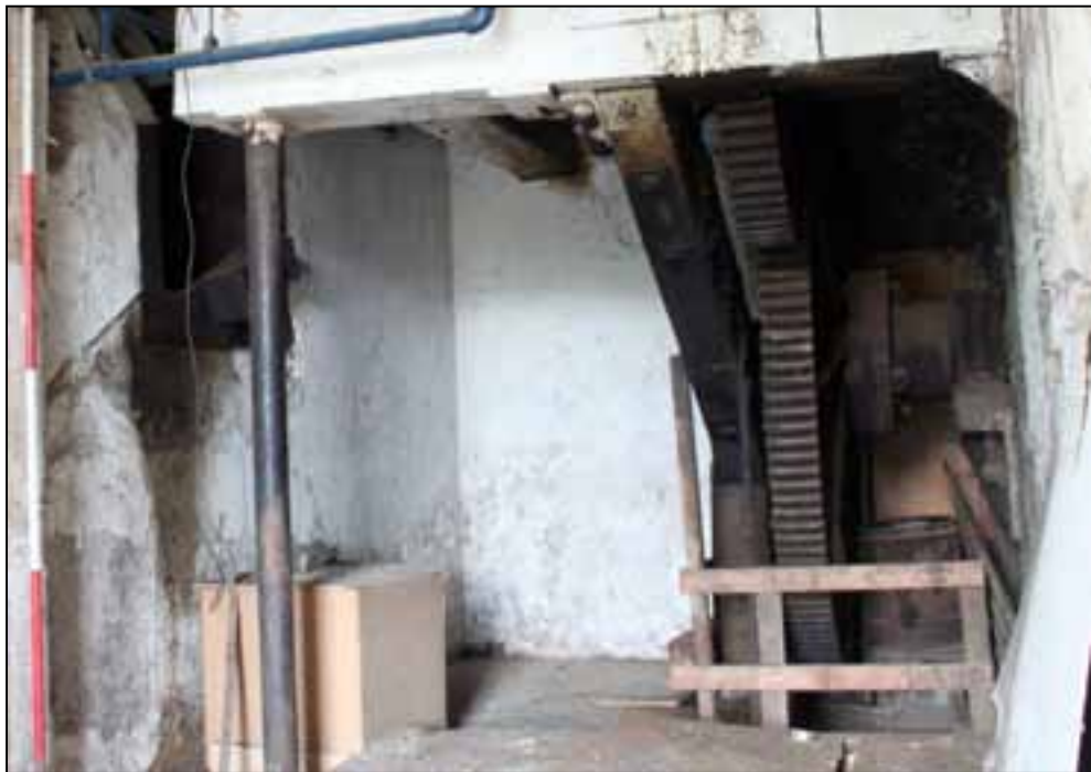
Plate 57: Extant waterwheel gearing
