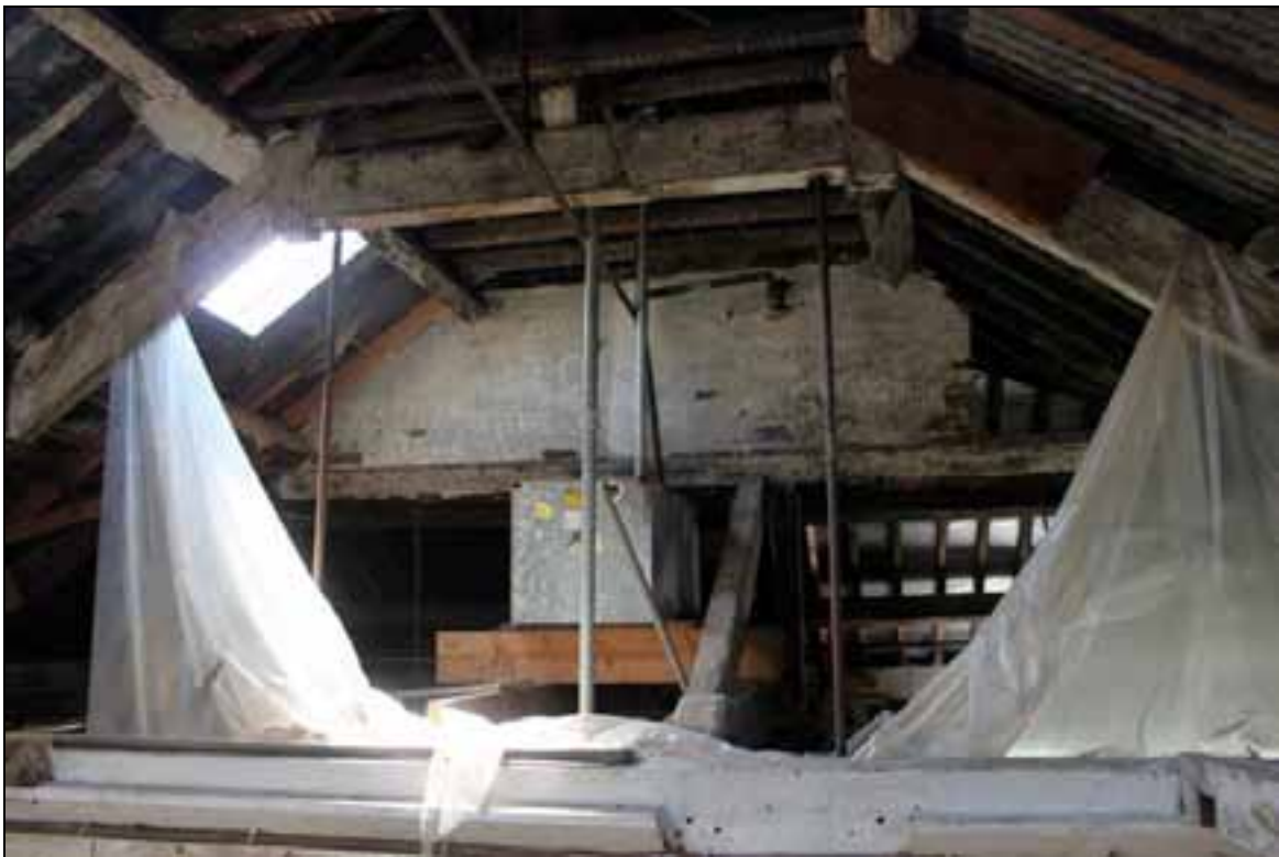
Plate 87: Lath and plaster partition between roofs of main mill and west wing, and queen post truss with replacement iron rods
