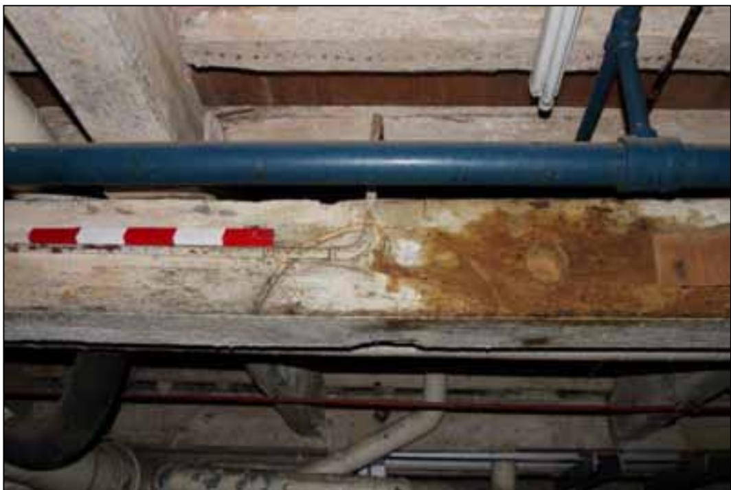
Plate 43: Scar of line shaft drum on face of beam
