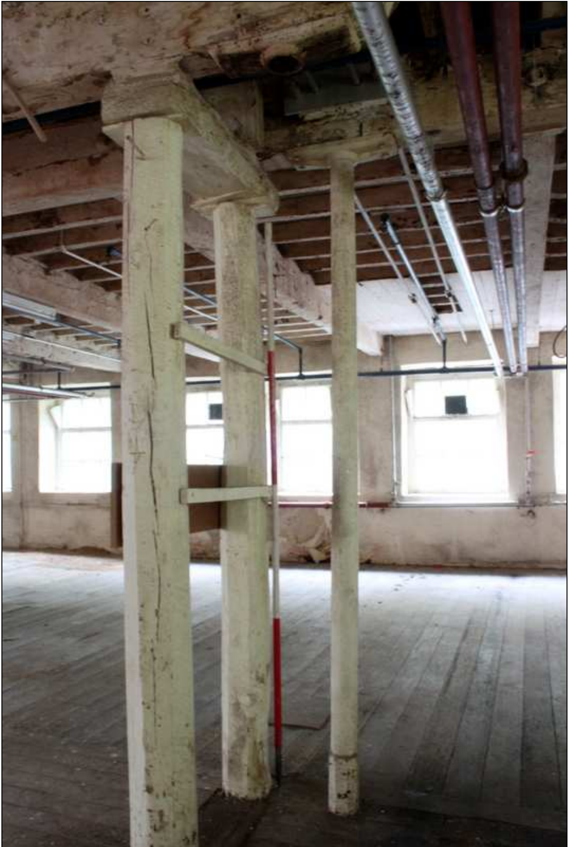
Plate 50: Timber props to ceiling beams adjacent to cast-iron column to scarf joint
