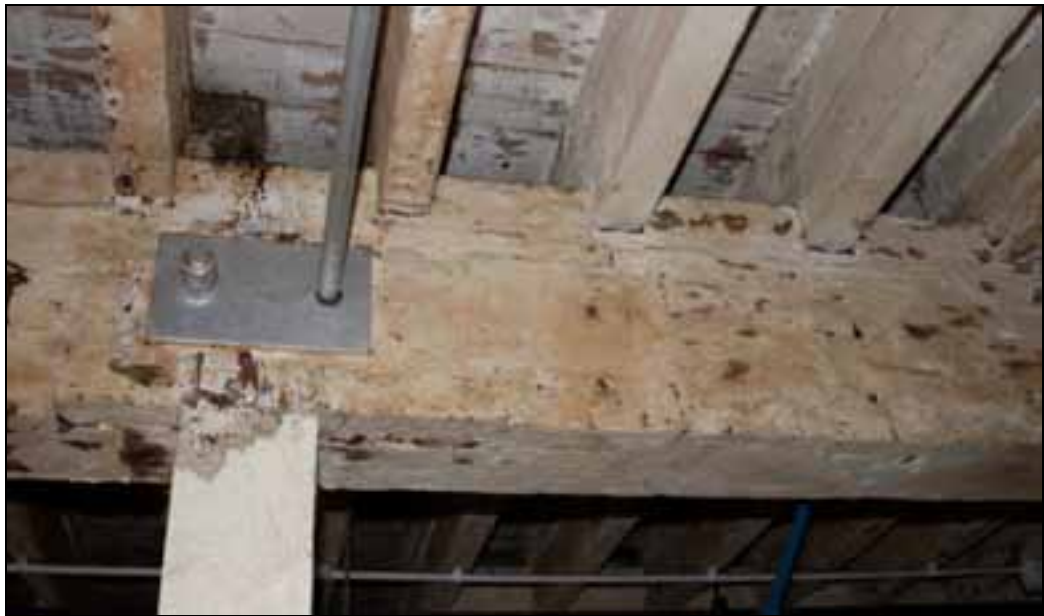
Plate 51: Timber fillet in beam face and later line shaft hanger bolt holes
