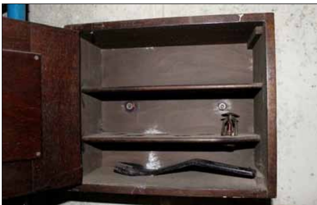
Plate 63: Cabinet housing spare parts for sprinkler system
