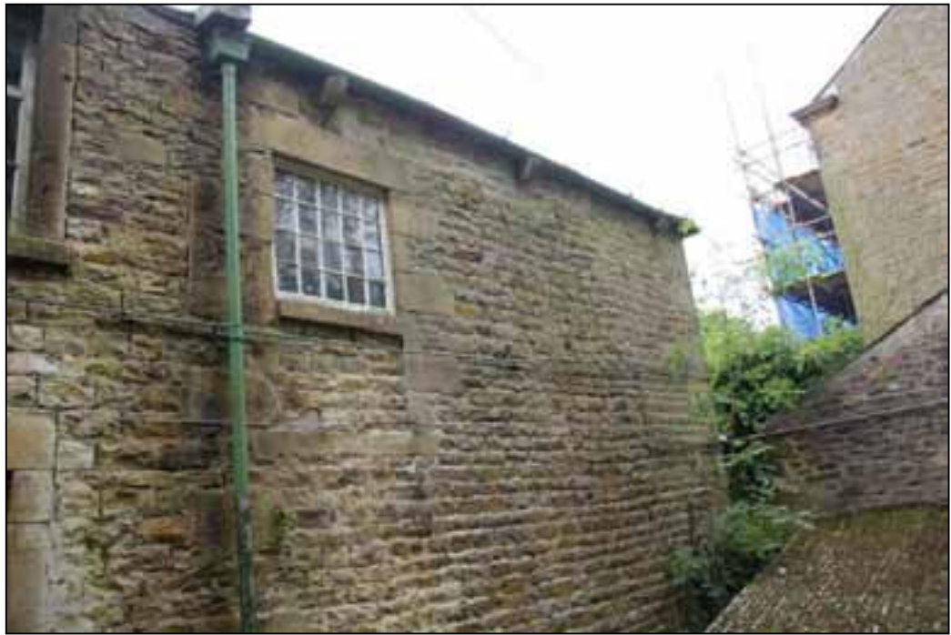
Plate 13: Butt joint between the west wing and the north wall, with blocked doorway
