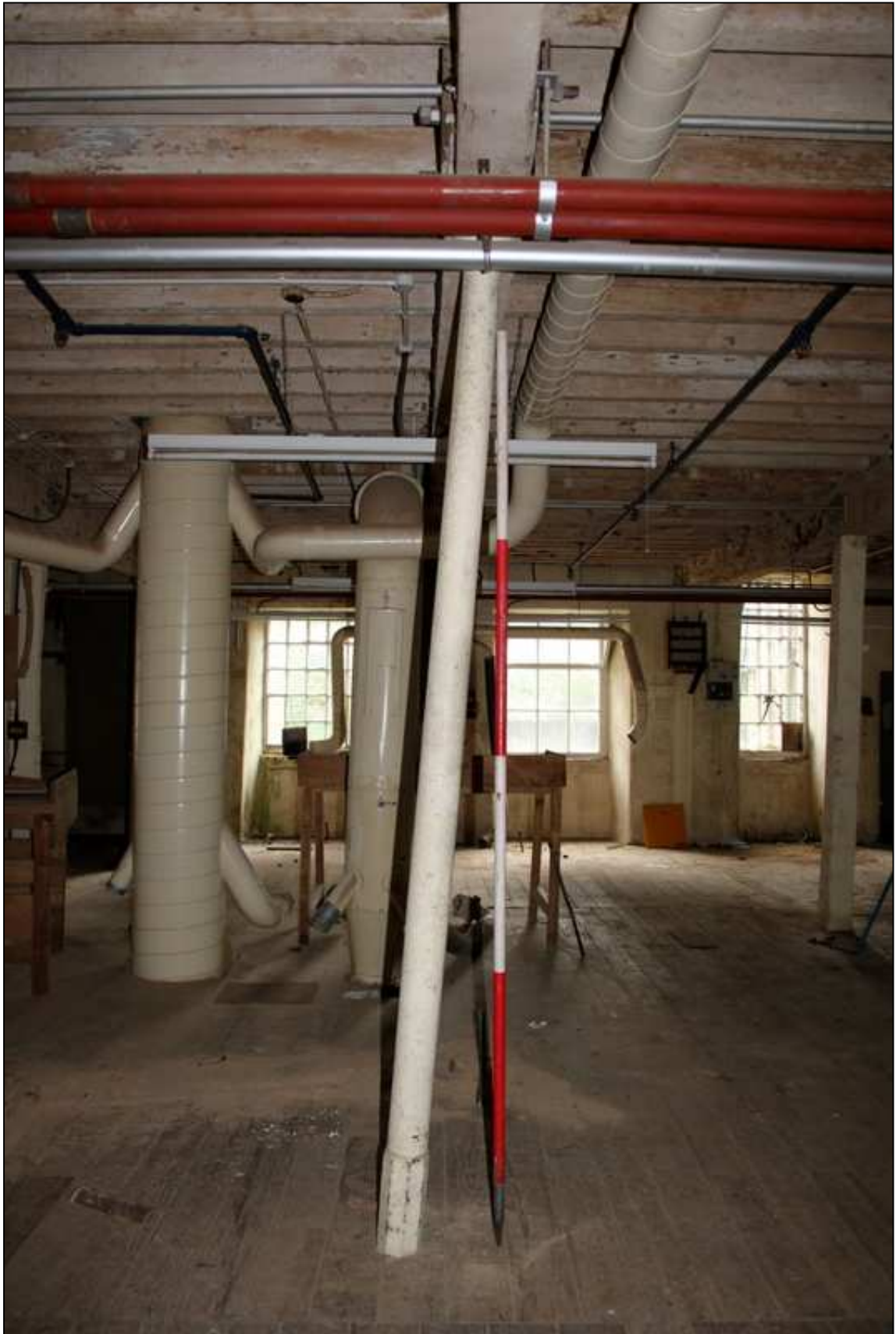
Plate 54: Deflection of first-floor column
