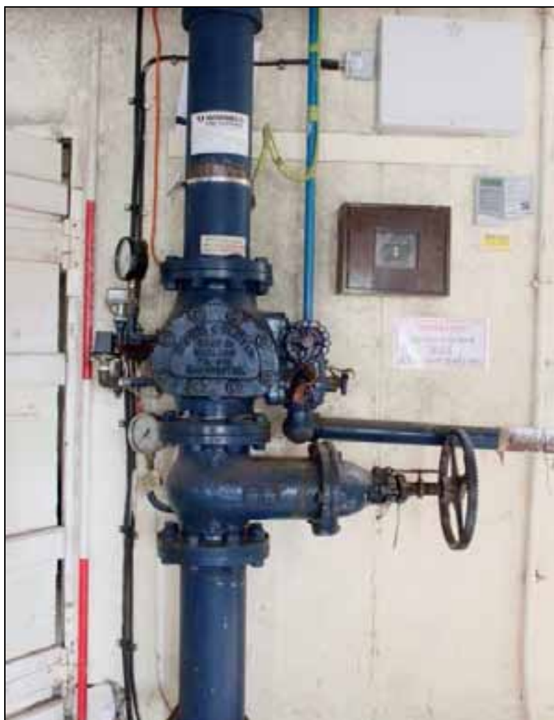
Plate 62: 'Christmas tree' control valve of sprinkler system
