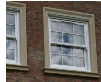
3. Reconstituted Stonework Window Surrounds
