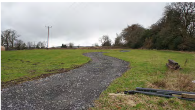
8 View from the middle of the development site looking north, showing the access track already constructed
