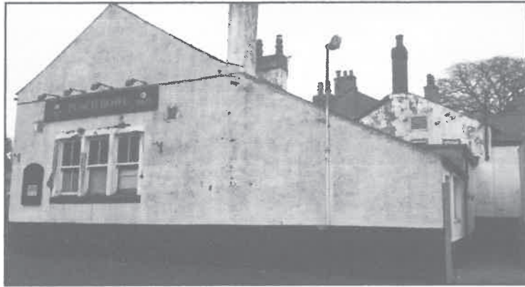
Figure 9) Western elevation of former barn range with catslide roof and rear outshut
