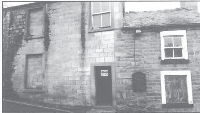
Figure 5) Eastern cottage (shown here to the right) with blocked door (behind notice board) and left hand later C19th addition (dwelling) at the eastern end of the building.
