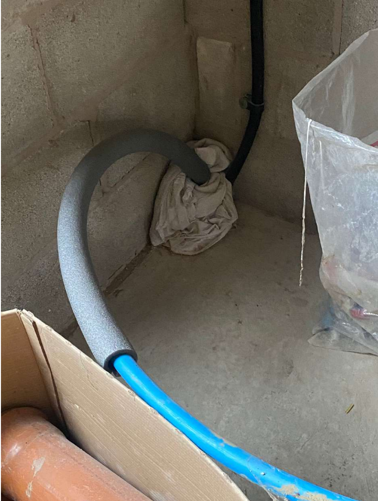
Plumbing as installed (blue pipe provides water connection)
