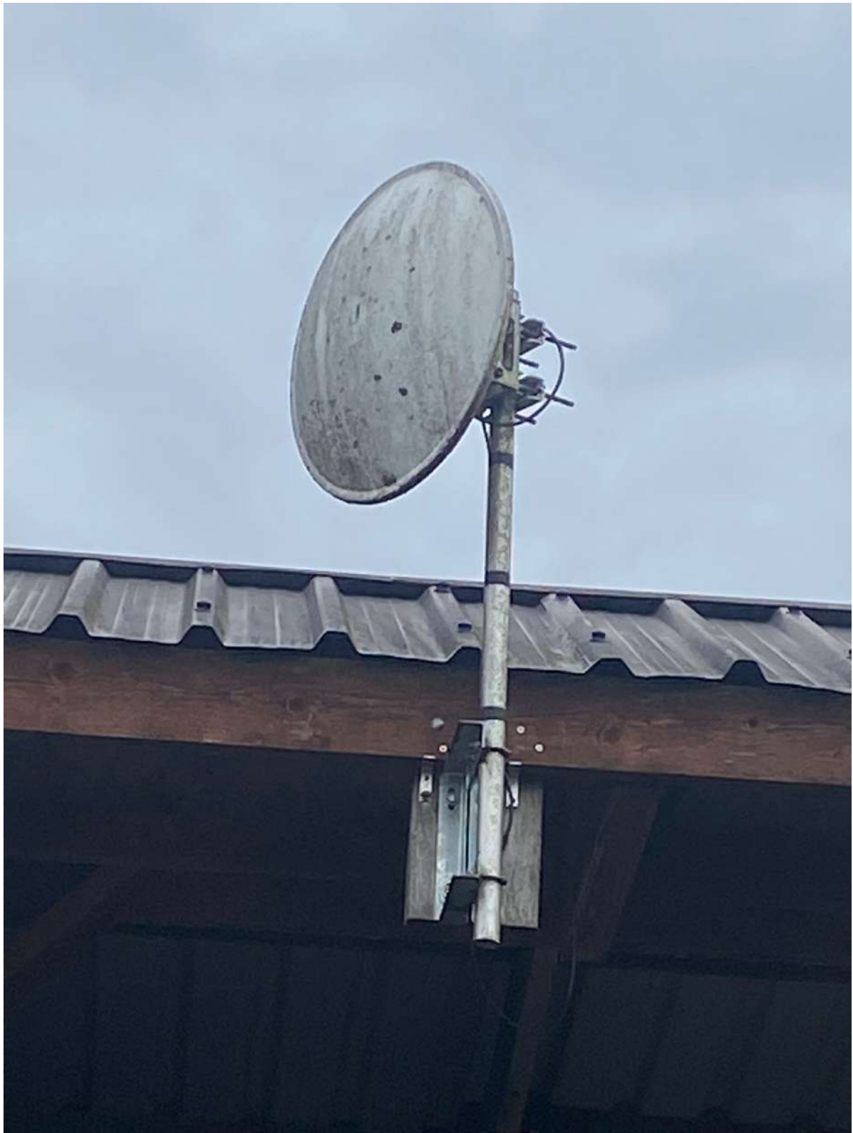
Satellite dish as installed
