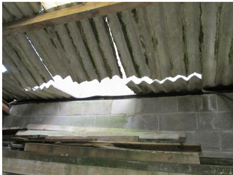
Photo 14 – Building A – Damaged Roof Sheet
