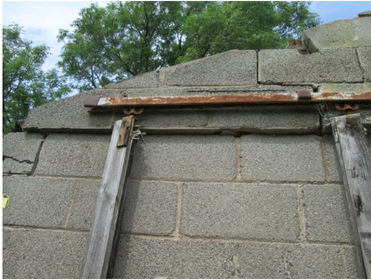
Photo 15 – Building A – Damaged Wall
