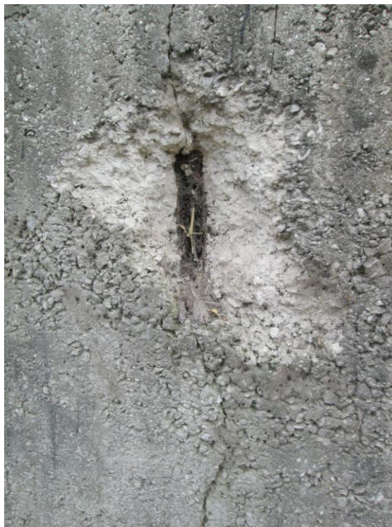
Photo 16 – Building B – Spalled Concrete
