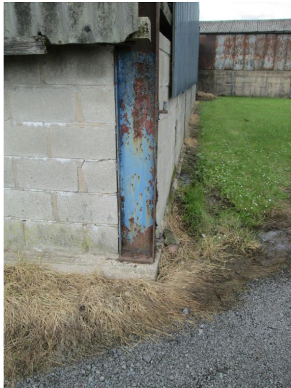
Photo 16 – Building C – Corroding Steel
