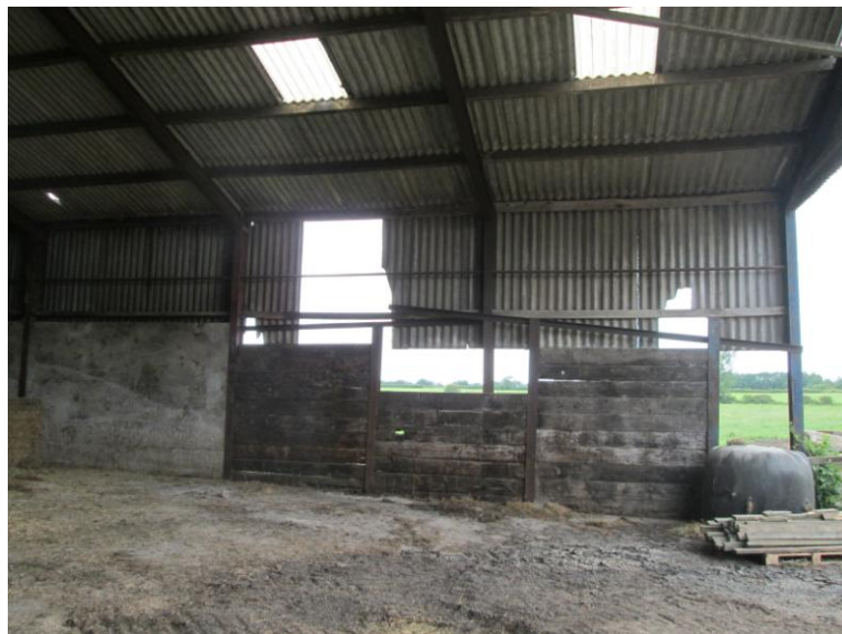
Photo 18 – Building C – Missing Wall Sheet
