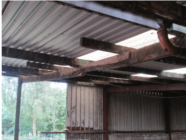
Photo 17 – Building C – Damaged Timber Rafter
