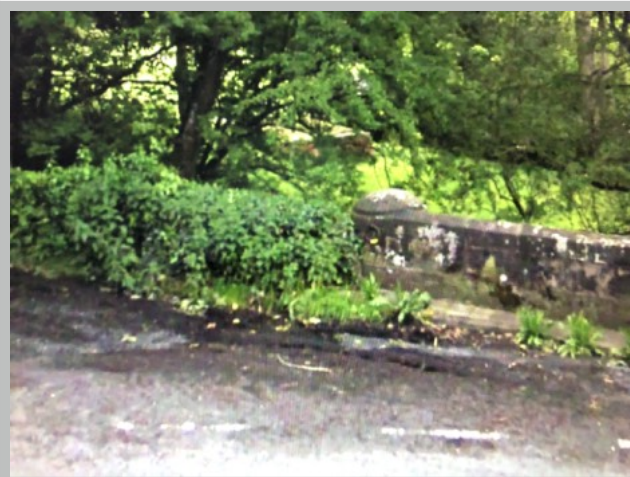
Plate 43a Hodder Higher Bridge and wall (owned by LCC) and as previously ivy-covered
