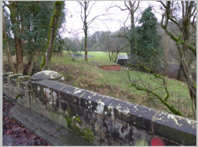
Plate 53. Pier at termination of S parapet and view into site in December
