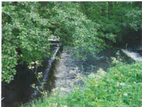
(ix) Upstream weirs opposite Talbot Hotel ISIS Unit: Broad Nosed Broad Crested Weir (used to represent the two upstream (of three no.) weirs)
