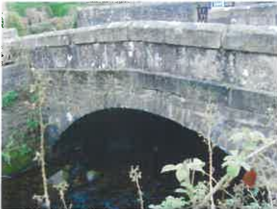
(iii) Malt Kiln Brow Road Bridge over Chipping Brook – upstream face ISIS Unit: Arch Bridge
