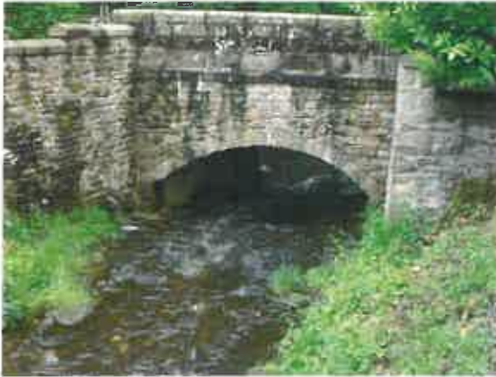
(i) Malt Kiln Brow Road Bridge over Dobsons Brook – upstream face Not explicitly modelled as it has sufficient capacity to convey all design event flows.
