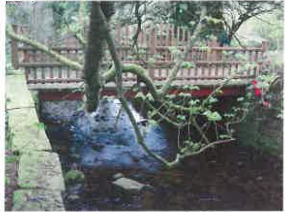
(ii) Mill timber access Bridge – downstream face ISIS Unit: USBPR Flat Soffit Bridge
