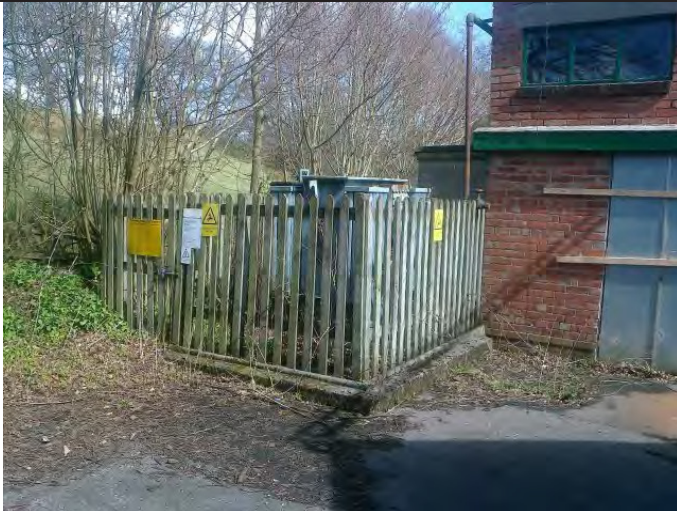
Photograph 11 (facing E): Electricity substation on the northern boundary of Area 1.
