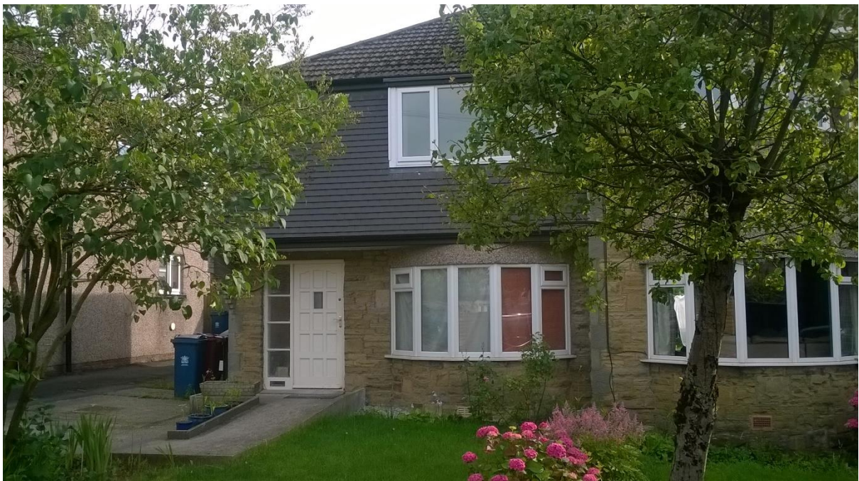
G. The original concrete tiles on some properties in the area are beginning to fail and are slowly being replaced. This example is 9 Warwick Drive.
