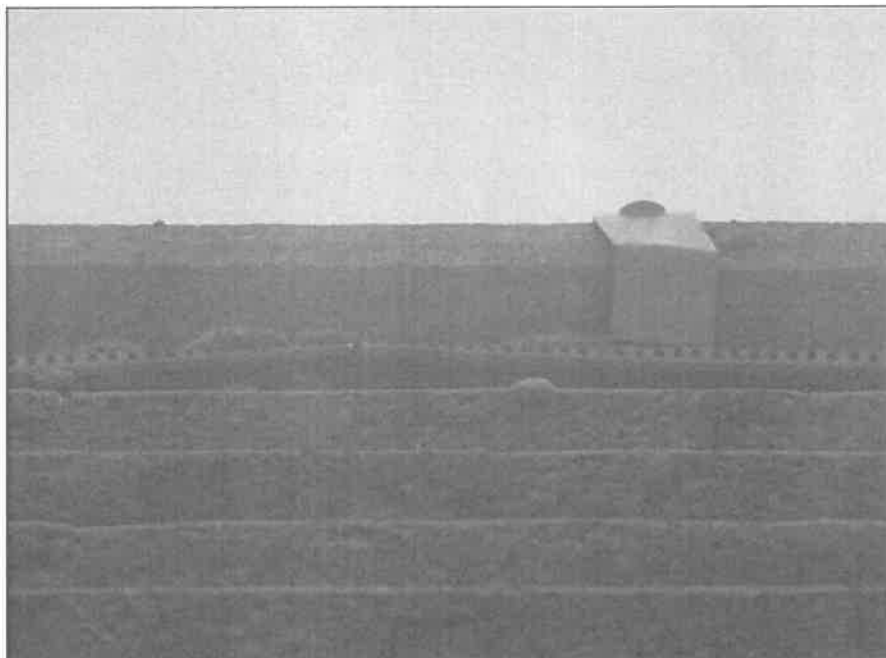
Plate 9: In places the ventilation was lifted enough for bats to easily gain access into the loft space.
