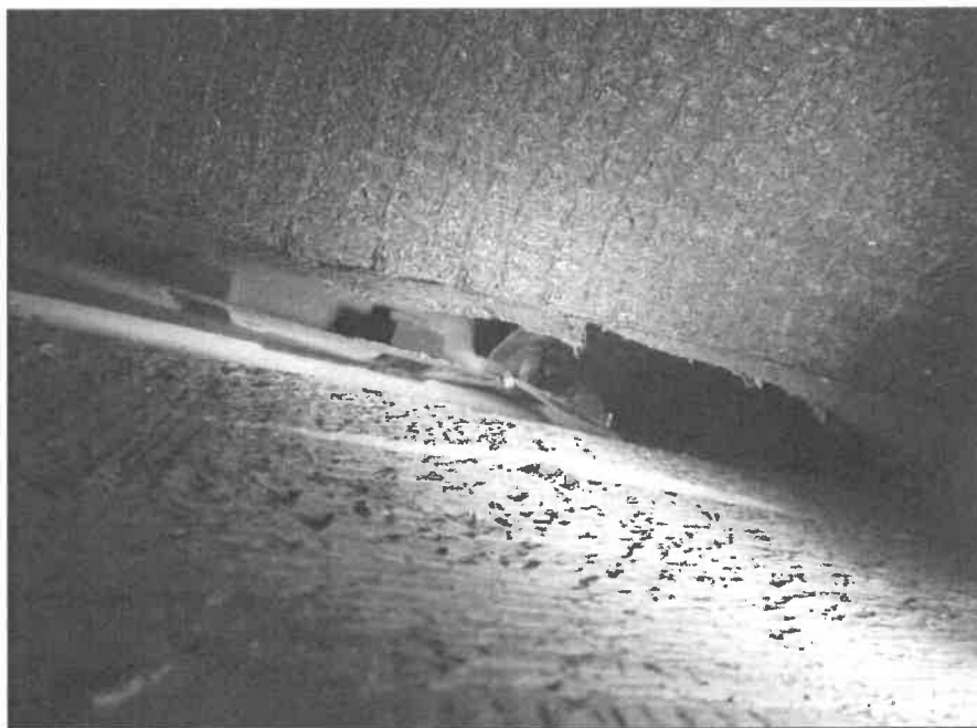
Plate 12: Within the gap, the plastic roof vent was visible.
