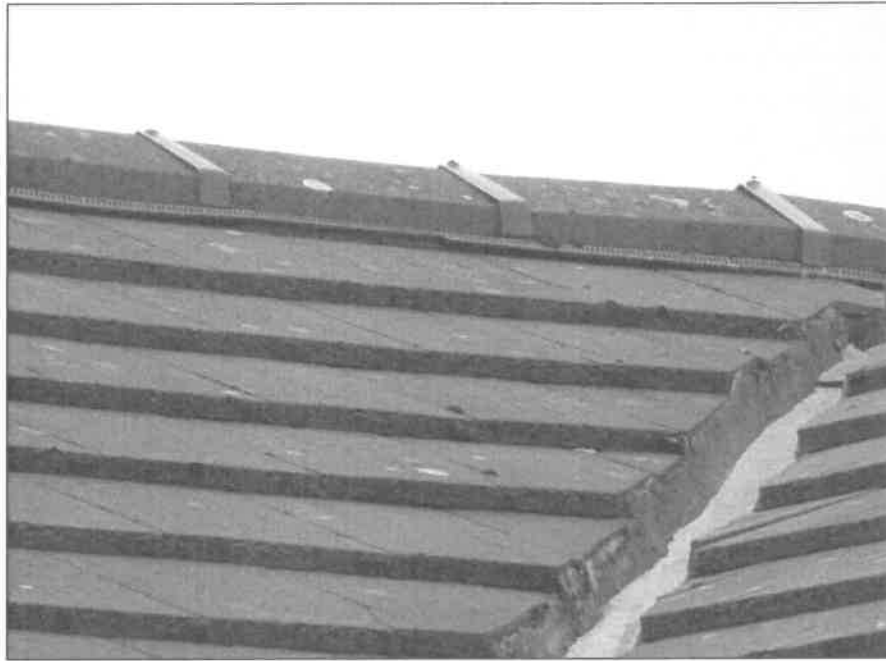
Plate 8: The plastic roof ventilation was lifted along the ridge tiles at the southern end of the property.
