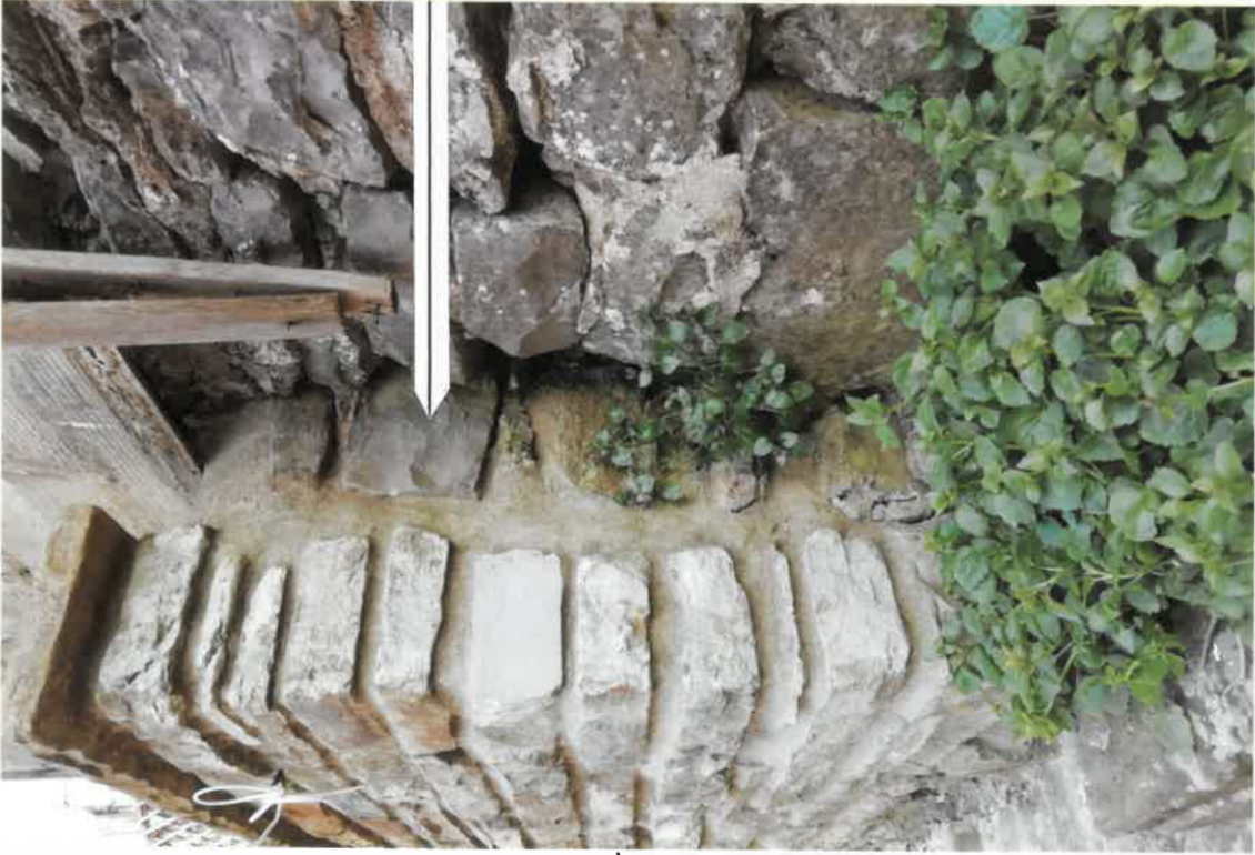
A. Outside wall of former coal shed of 2 Sawley Rd B. Fascia recently built
