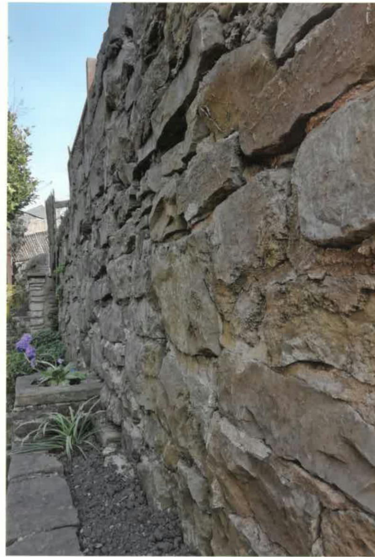
Rear of modern outbuilding's façade built on top of 45cm wide dressed sandstone boundary wall
