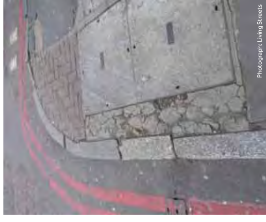
Poor quality pavement
