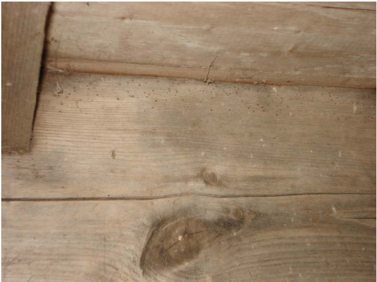
Plate 17 – Wood boring insect infestation to first floor beam (Stalls)
