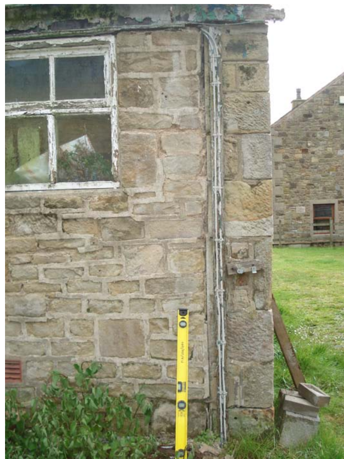
Plate 10 – Butt joint @ Store 6 front/gable elevations
