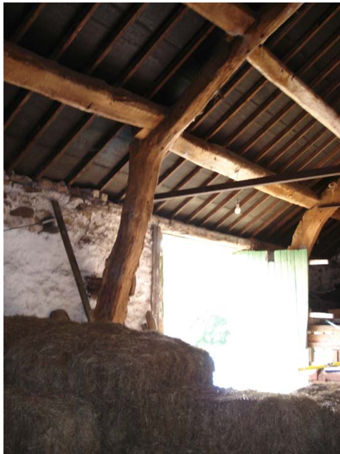
Plate 21 – 'Cruck' frame historic deterioration/section reduction
