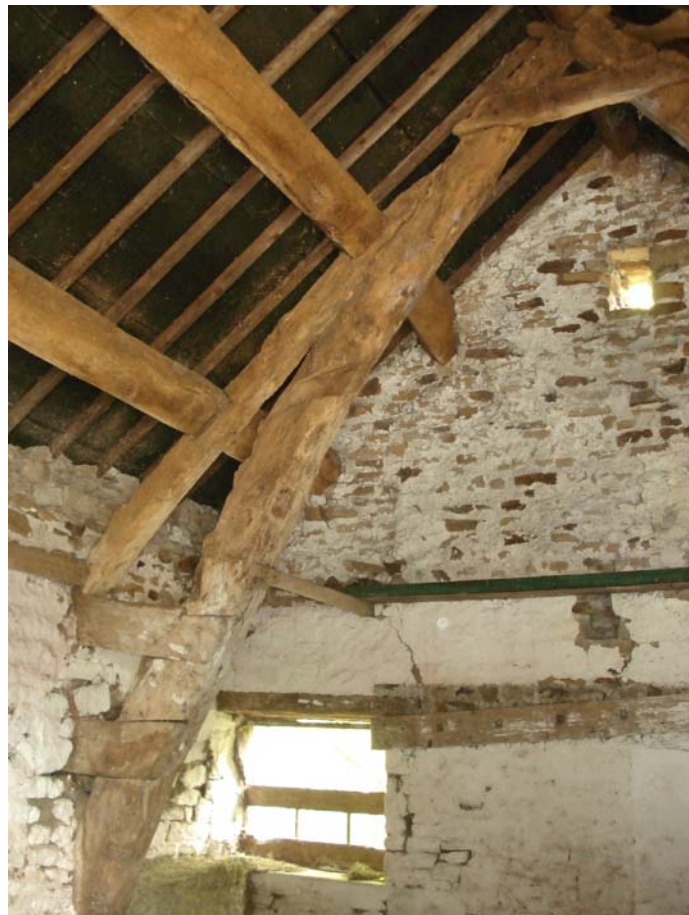
Plate 20 – 'Cruck' frame historic deterioration/section reduction
