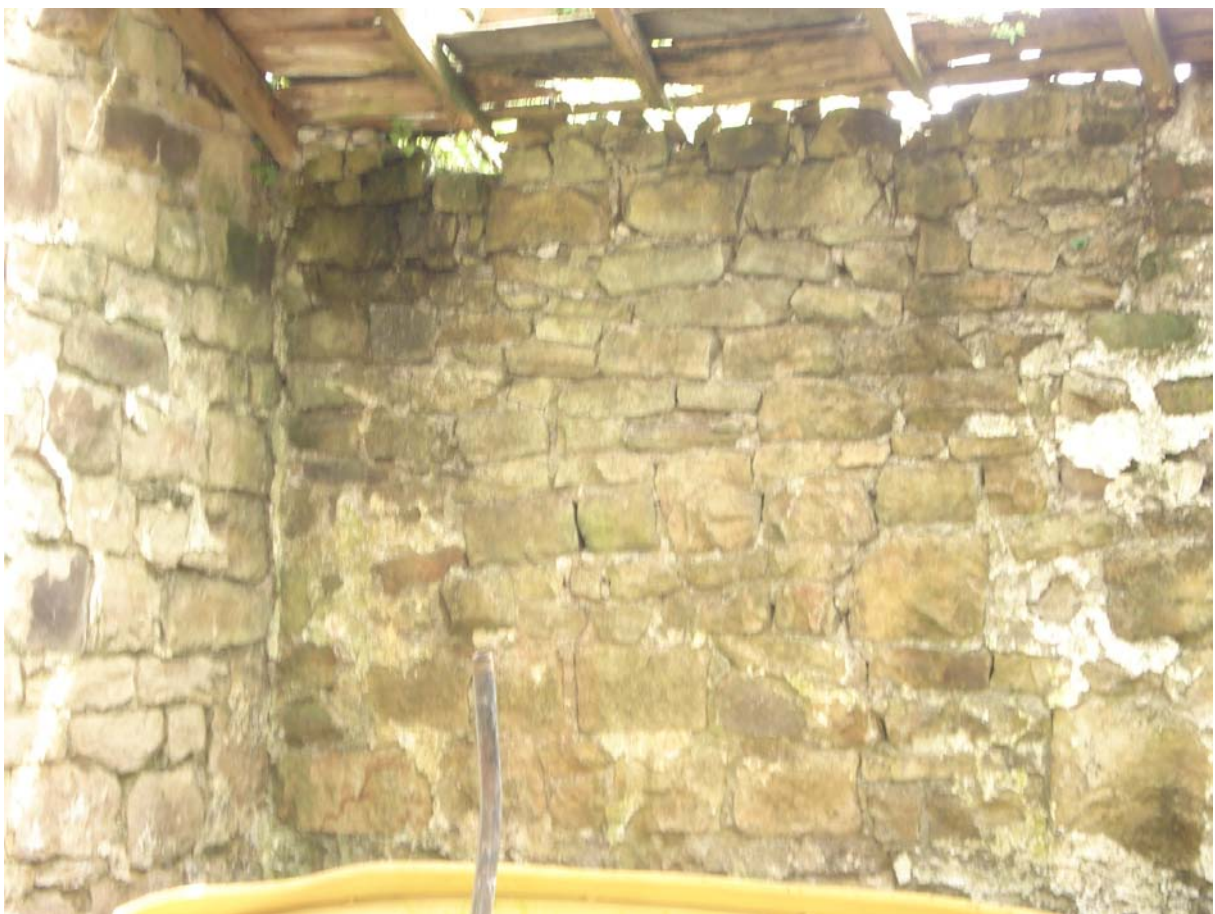
Plate 34 – Store 5 rear elevation – weathered mortar bed and perpend joints
