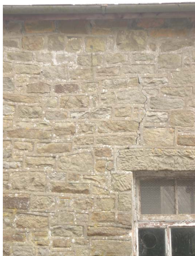
Plate 04 – Vertical cracking at lintel bearing within Barn rear elevation
