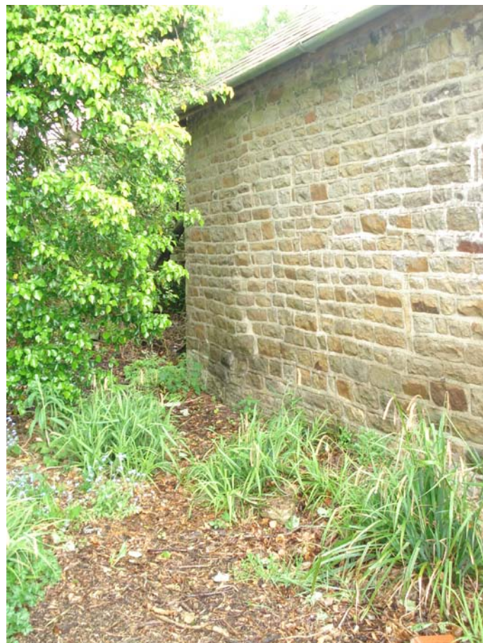
Plate 02 – 'Bulge' within rear elevation adjacent to northern gable
