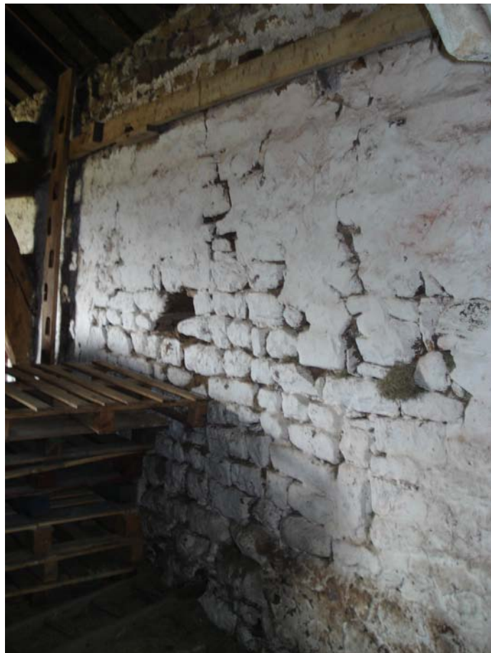
Plate 22 – Spalled mortar within internal aspect of Main Barn
