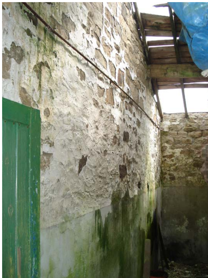
Plate 36 – Spalled whitewash finish to Store 5/6 partition
