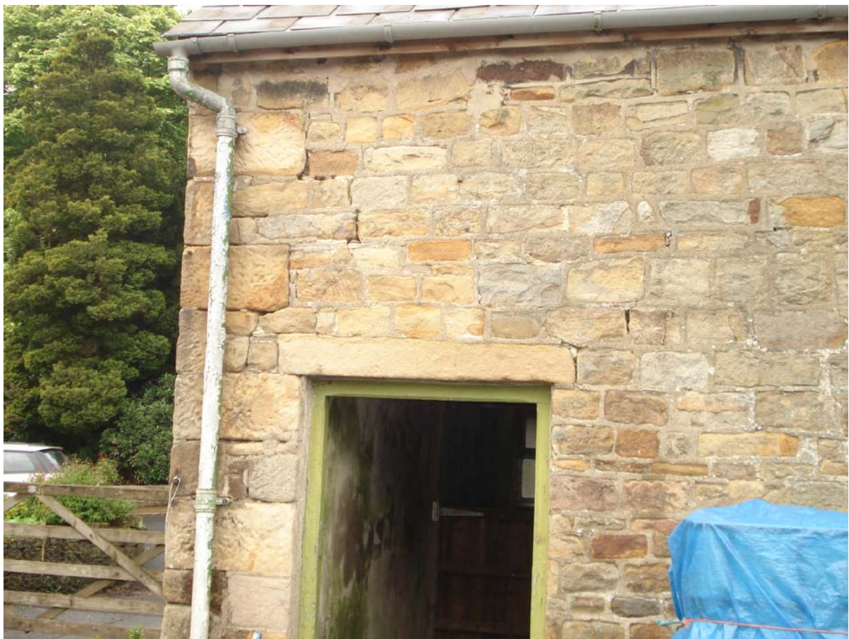
Plate 07 – Historic movement/visible cracking within Barn front elevation
