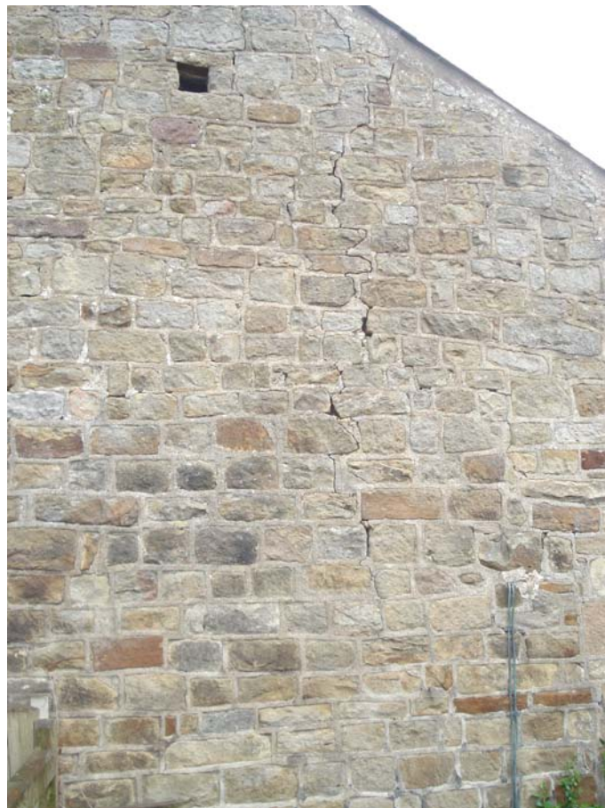
Plate 06 – Vertical cracking within Barn gable elevation
