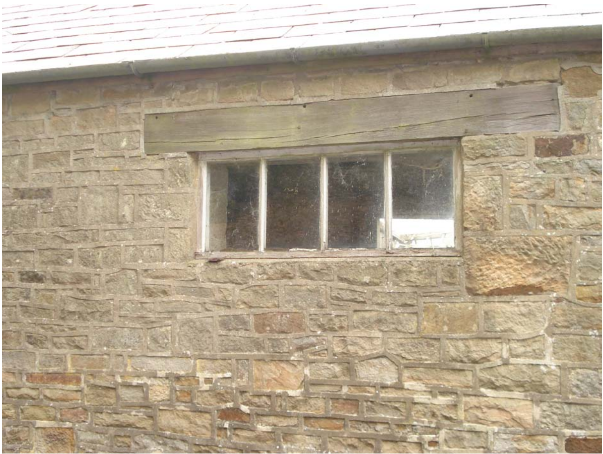
Plate 03 – Thermal cracking to timber lintel within Barn rear elevation
