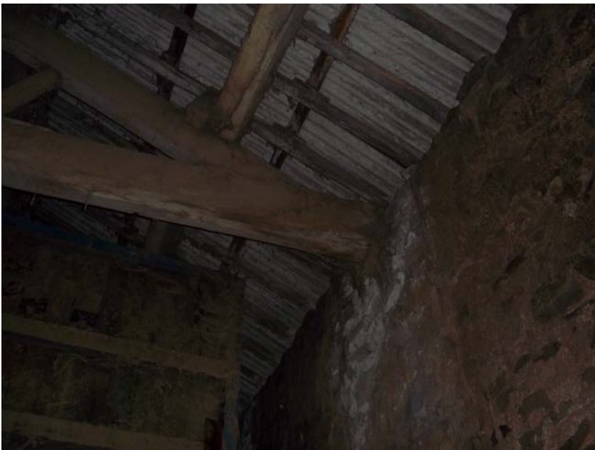
Internal Truss Support Deterioration of Truss End Bulging to Wall
