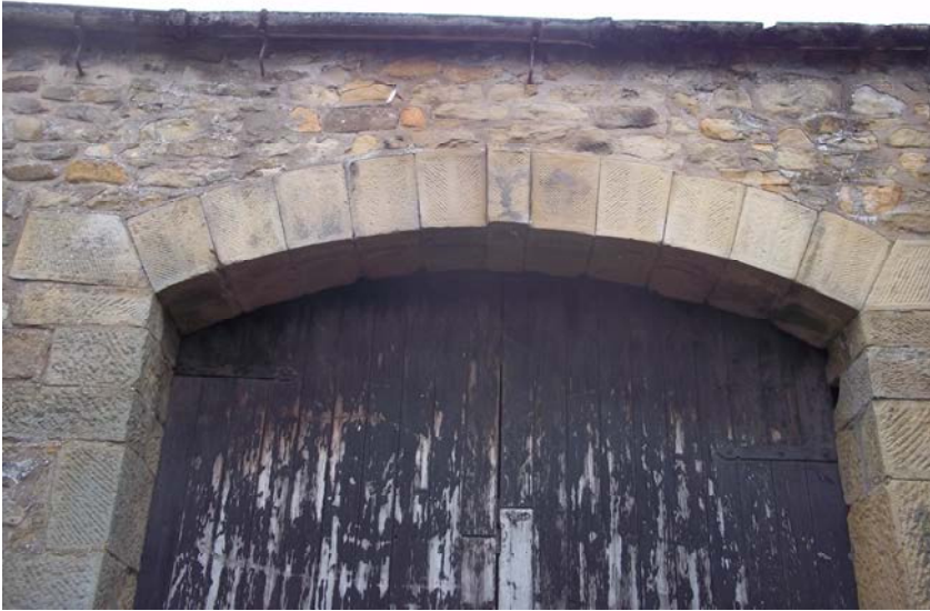
Right Hand Doorway Cracking to Right Hand Side
