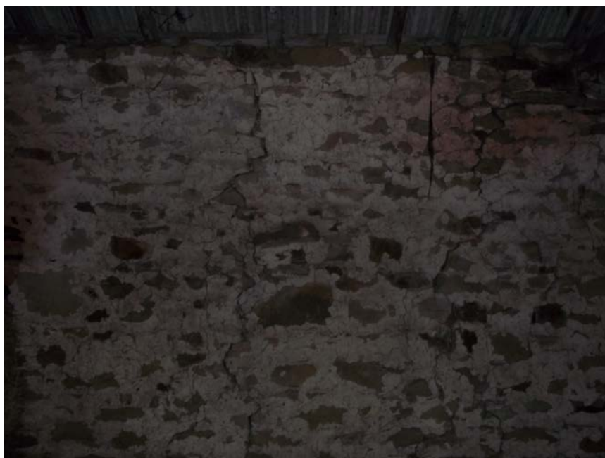
Cracking to Internal Wall
