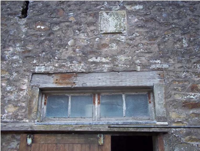
Front Elevation Cracking over Door
