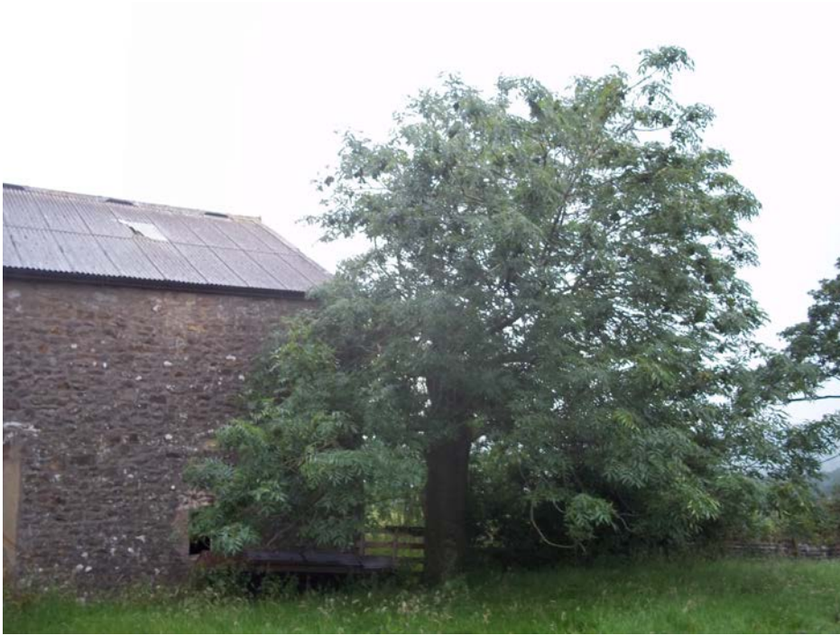
Rear Left Hand Corner Showing proximity of tree
